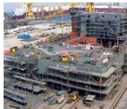
More than half of the structural fabrication work have been completed for the liftboat, which is expected to be fully constructed by end 2015
