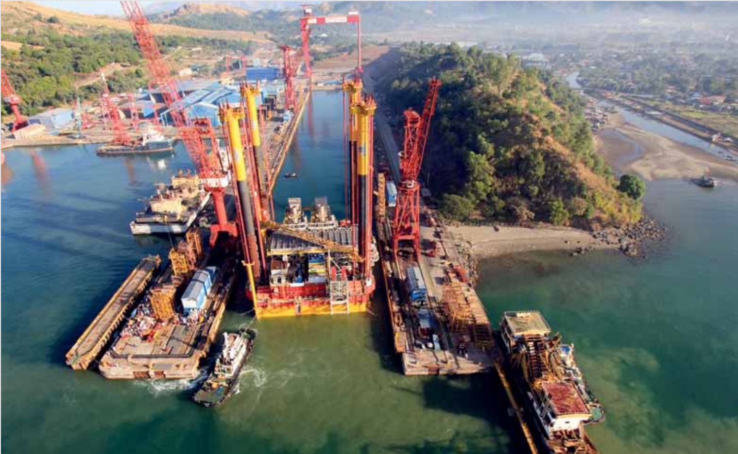
The Depletion Compression Platform (DCP) being towed out of Keppel Subic Shipyard's dock to its handover site
