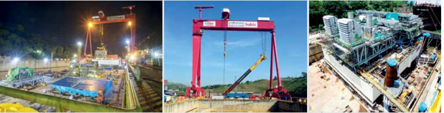
(From left) Lifting of the air cooler module; The 1,500-tonne gantry crane lifting the 62-metre long upper section of the tubular leg to an upright position; Integration of the modules after the completion of the lifting campaigns
