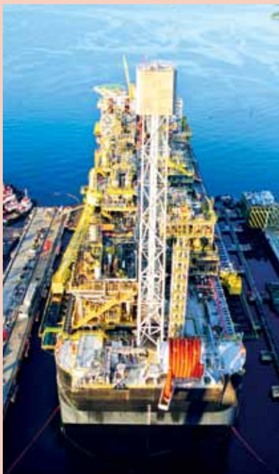
Lifting operations for the installation of topside modules and flare tower for P-66 progressed smoothly
