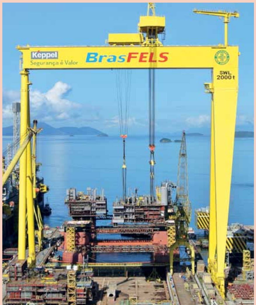
Installation of upper hull modules has commenced for the second DSS™ 38E semisubmersible rig Keppel is building for Sete Brasil
